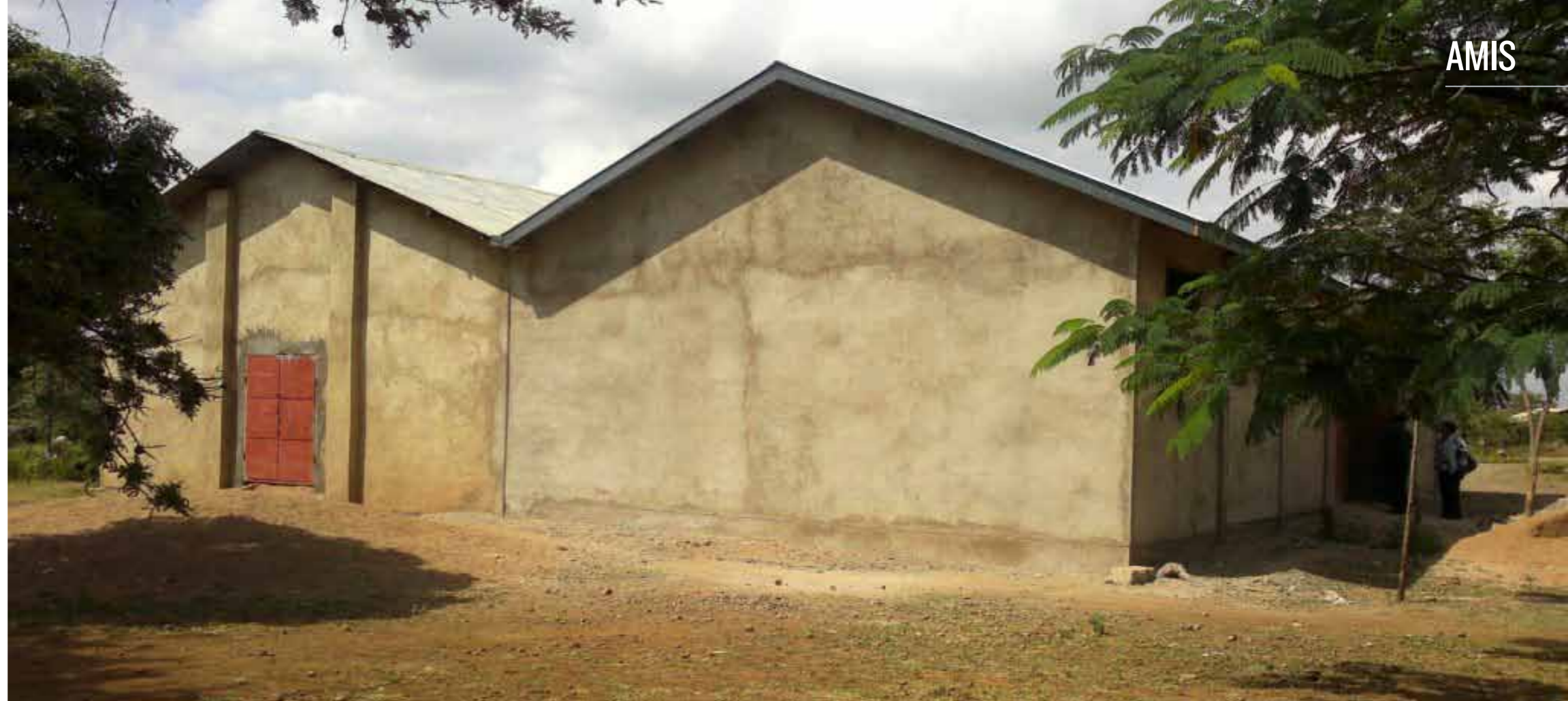
Malula grain storage warehouse located at Malula near Arusha, Tanzania, after being refurbished to a working standard
