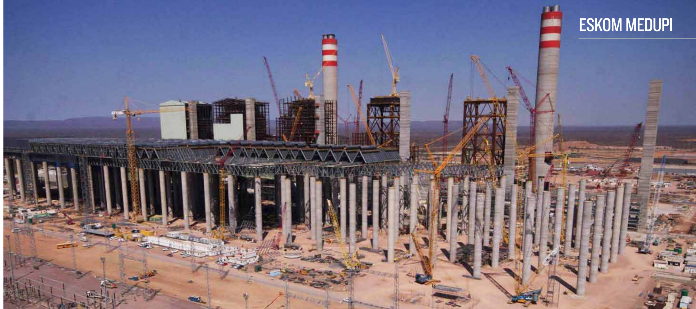
High voltage yard, air cooled condenser columns with boiler units and two chimneys
