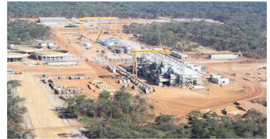
Sentinel plant area
