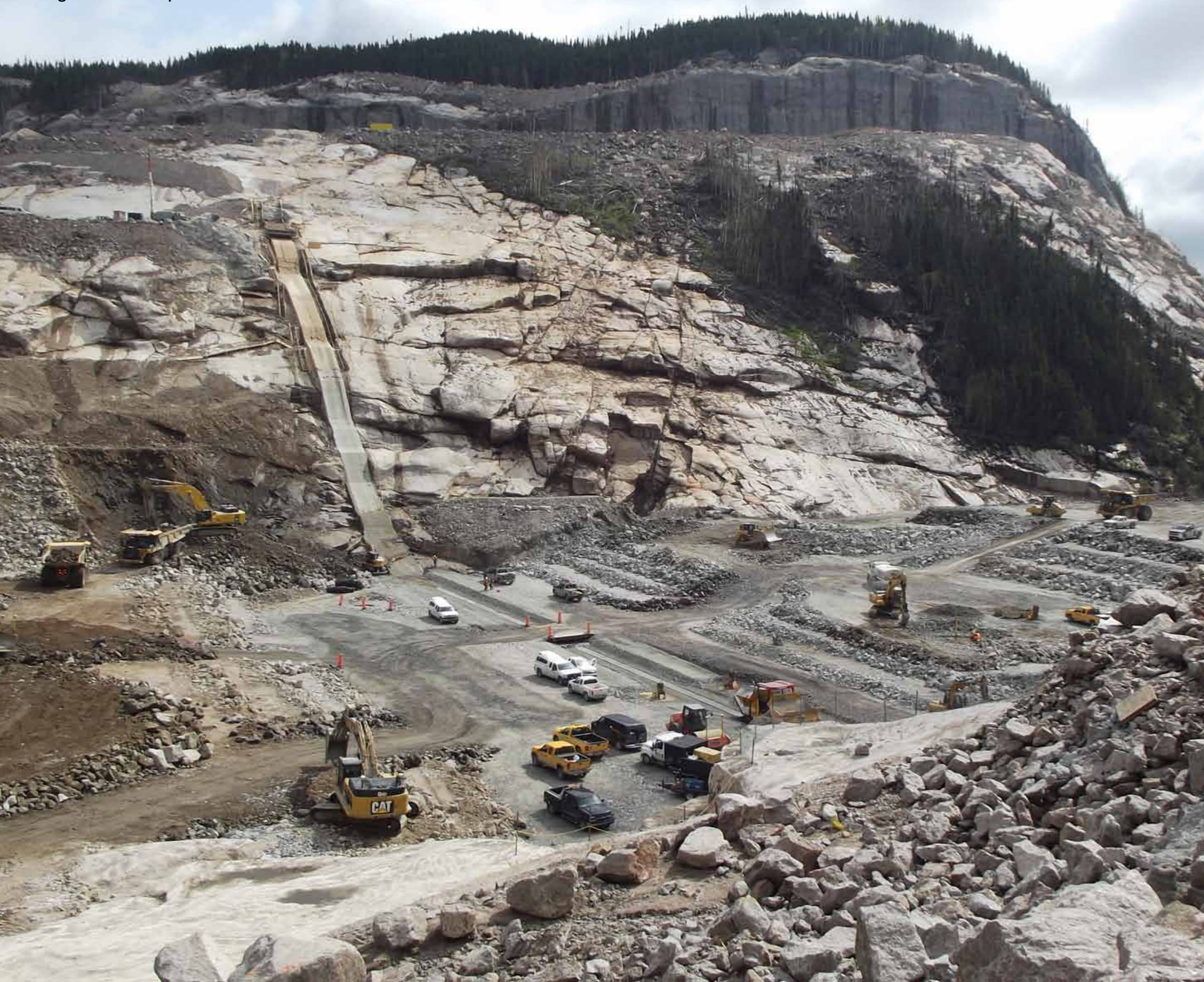
A view of the dam as the ground work begins to take shape
