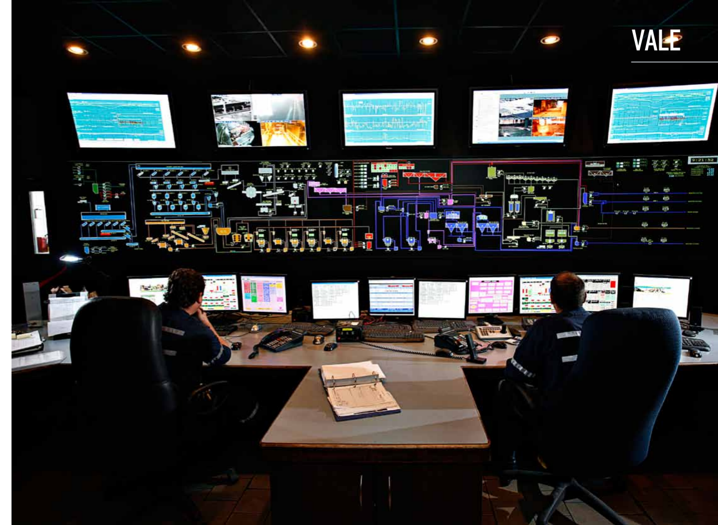
Clarabelle Mill control room
